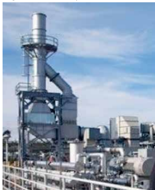
Figure 10 EBMUD's gas turbine cogeneration facility 32 .
